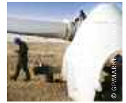
image MAINTENANCE WORKERS FIX THE BLADES OF A WINDMILL AT GUAZHOU WIND FARM NEAR YUMEN IN GANSU PROVINCE, CHINA.
