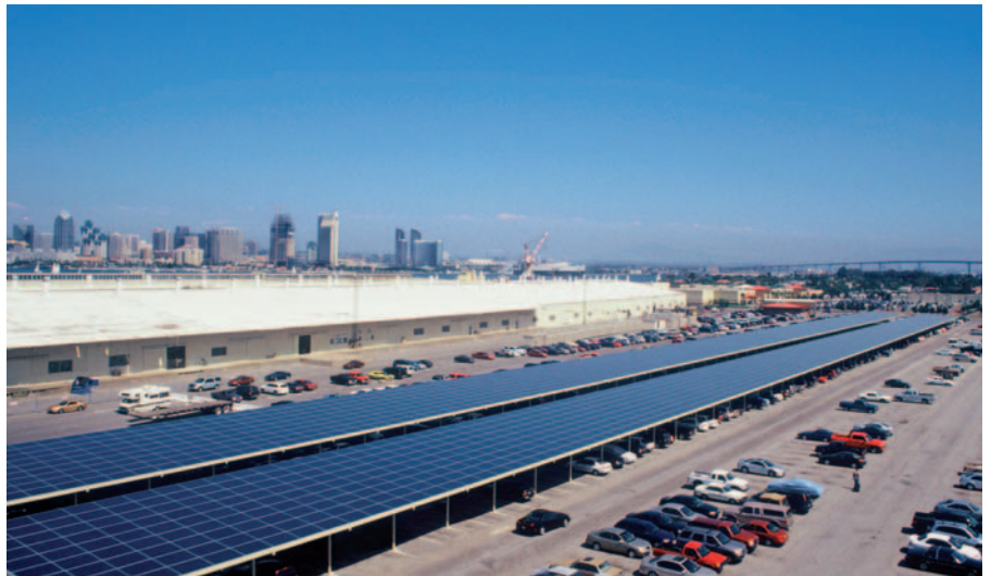
A 750-kilowatt solar-photovoltaic installation at a US Navy base in San Diego.
